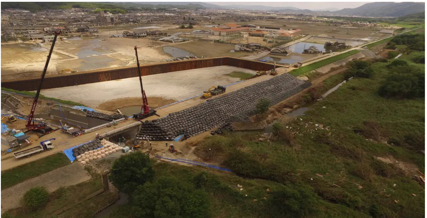
PICTURE 1: The temporary levee (source: MLIT Mabi Bureau)
